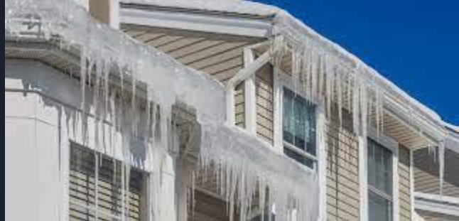
Ice Damming- Lack of ventilation
